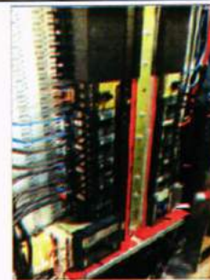
Vista de Panel principal
