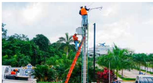
First camera of the Monitoring Center
